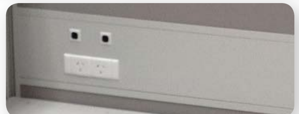
Soft-wired Cable Duct
